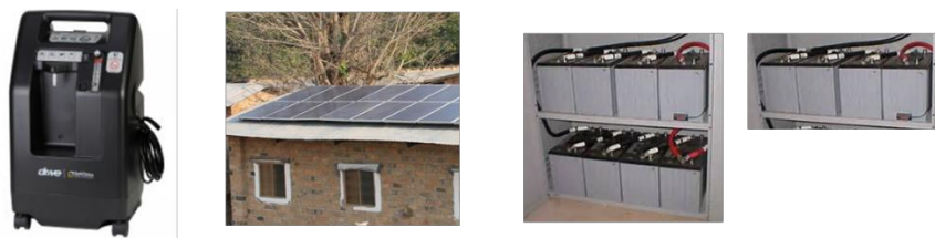
Figure 2. Solar power system for medical oxygen in Shamwana hospital after handover
