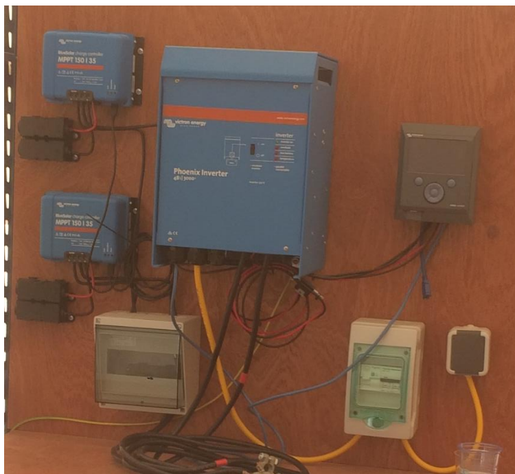
Figure 7 – Solar charge controllers, inverter and control panel for test setup.
